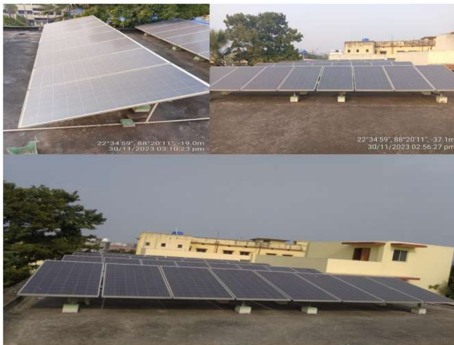
Figure 3.5: Rooftop Solar PV Renewable Energy Generation System
