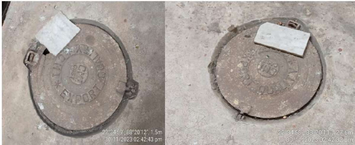
Figure 3.4: Rain Water Harvesting Tanks installed in the Campus
